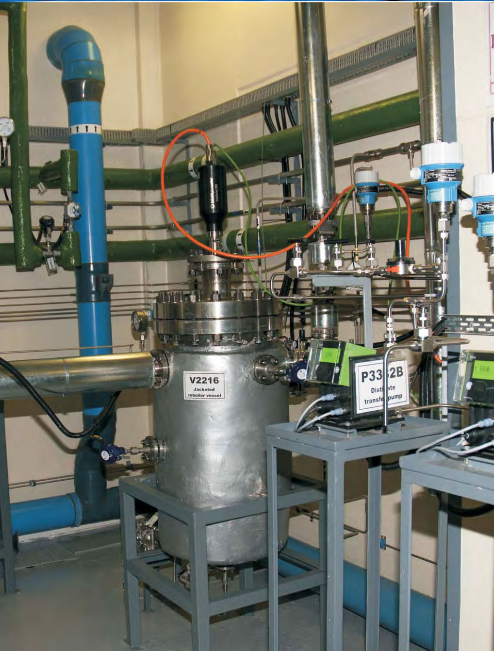
The MFPP distillation column at the Pelchem Fluorochemical Plant at NECSA
